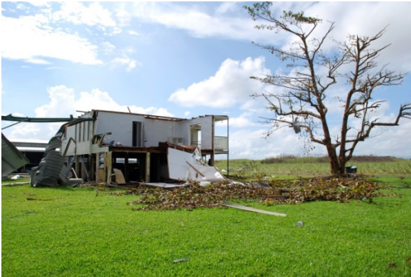
Figure 4: Example of damage to older house - Cyclone Yasi (Source: JCU CTS)
