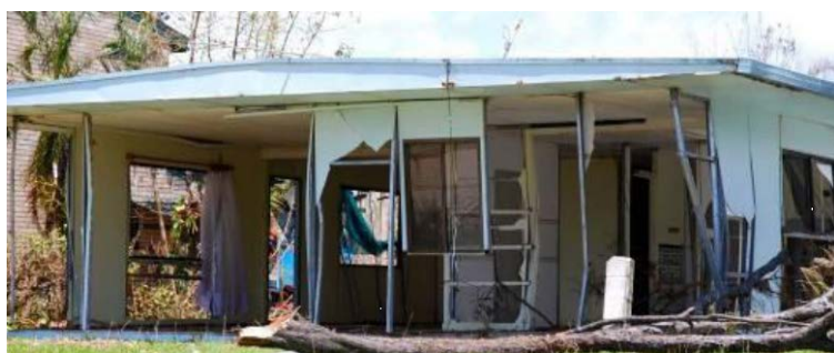
Figure 5: Example of storm surge damage– Cyclone Yasi (Source: JCU CTS)
